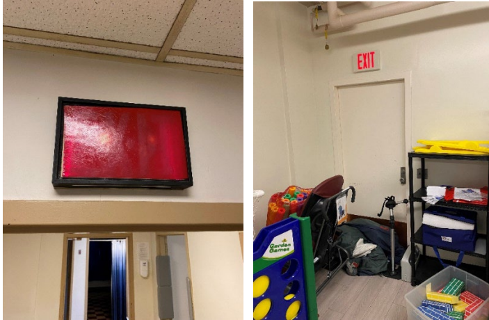
Photograph 3 (left): Non-illuminated exit sign.
