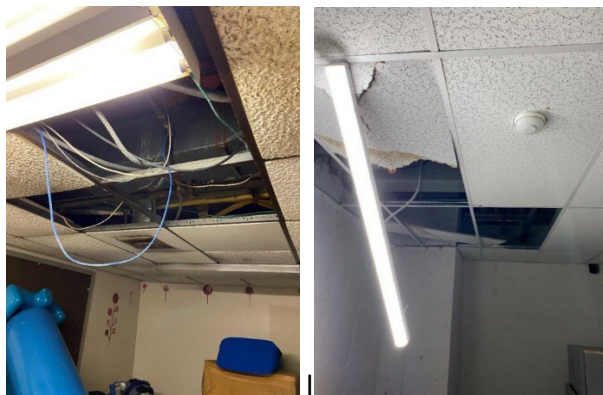
Photograph 1 (left): Missing ceiling tiles.
