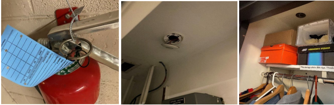
Photograph 5 (left): Fire extinguisher month inspection tag not filled out. Photograph 6 (center): Smoke detector not properly mounted. Photograph 7 (right): Obstructed sprinkler head.
