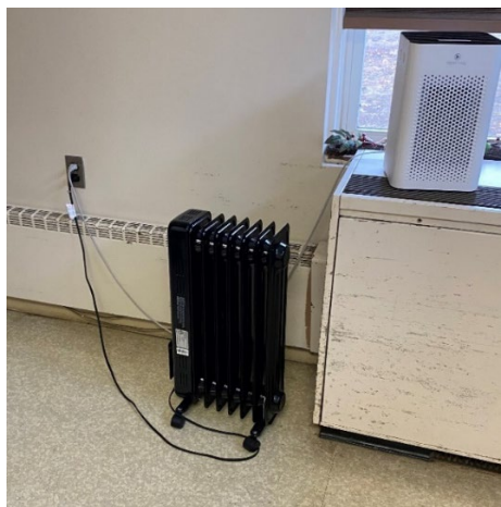
Photograph 9: Prohibited space heater in resident area.
