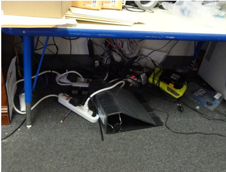
Photograph 1: Numerous electrical cords under a desk in an unlocked office that was accessible to children.
