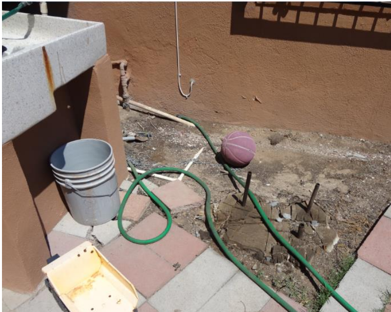
Photograph 10: Steel pipes poking out of the ground in an outside play area.
