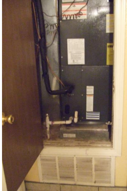
Photograph 7: Unlocked hallway door that led to the heating, ventilation, and air conditioning system, which had pipes and wires accessible to children.
